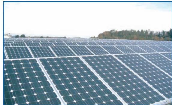
Photovoltaic system Petersen Alpa (Germany) planned on the basis of premium site audits during ENVISOLAR, source Enecolo
